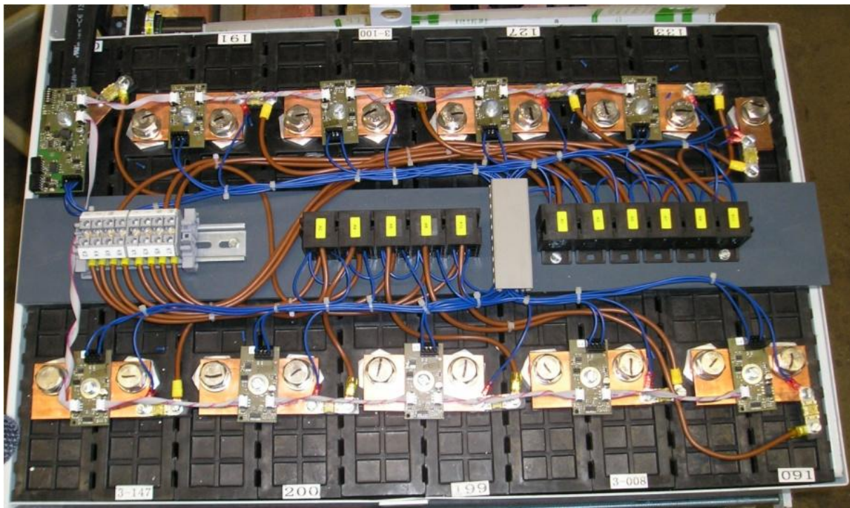
figure 1: Cluster of \text{LiFePO}_4 cells including monitoring- and balancing circuitry (with kind permission of R. Gross, BNO-consult, 97337 Dettelbach, Germany)
